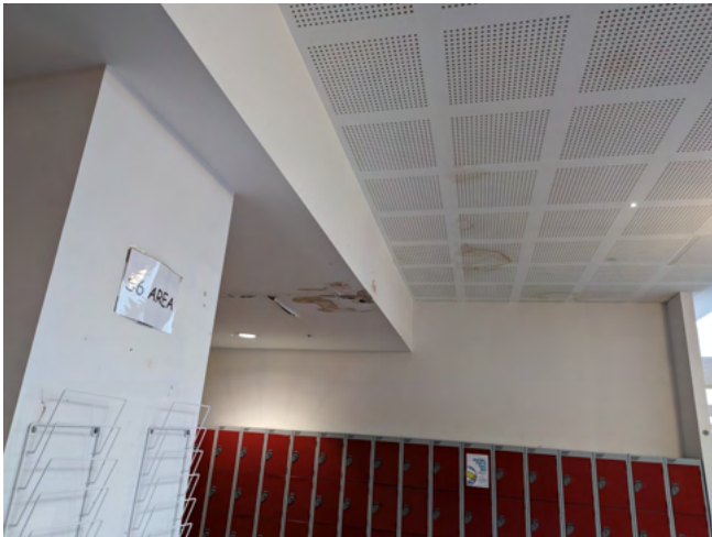
Example of water damage due to leaks (various issues over the year, only 9 years since new)
